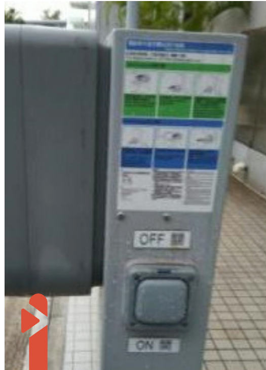
Installed outdoor at EMSD headquarters 在機電工程署停車場安裝
